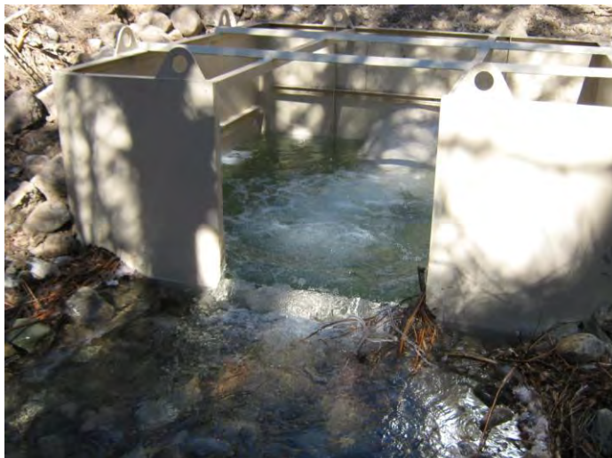
View of the dissipation box for the Acequias de Chamisal Y Ojito drop structure. This project was designed and inspected by Taos SWCD and funded with ARRA stimulus funds.
